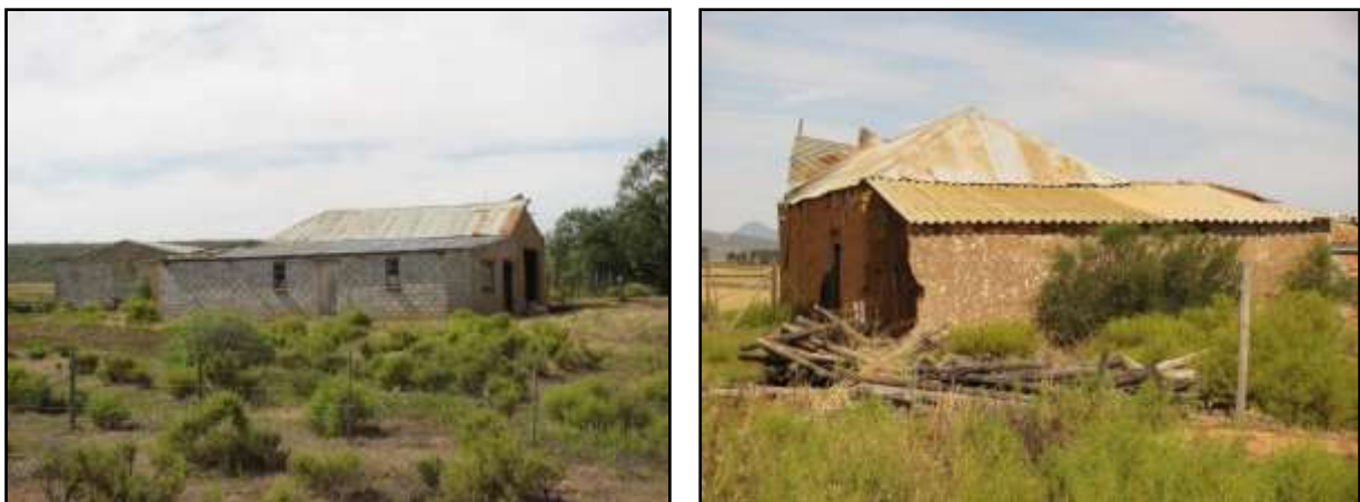
Plate 6 & 7: The transformed shed on Rossouwskraal comprising a collapsing, unfired mud-brick building with recent cement block additions.
