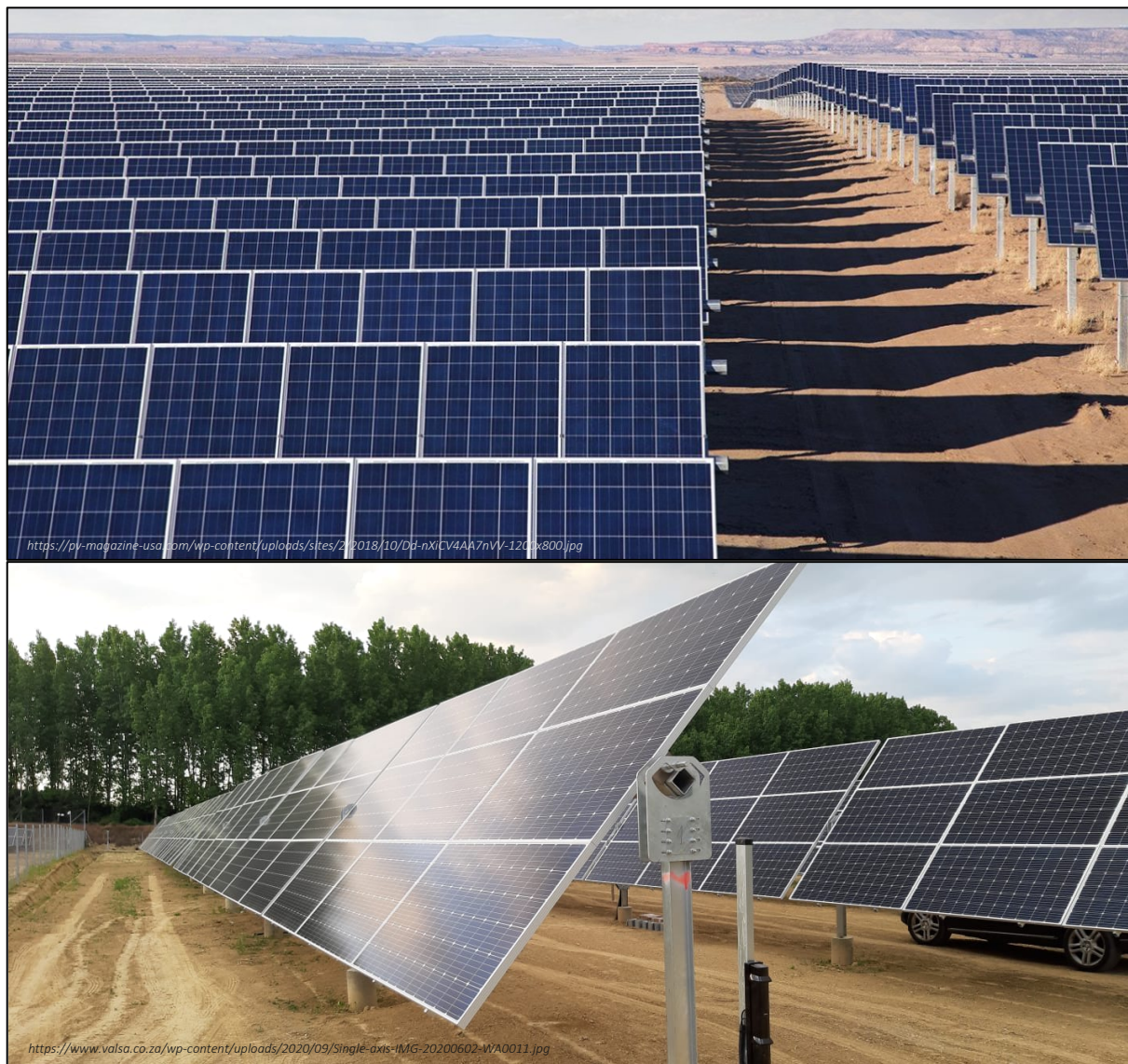
Figure 3.3 – Examples of installed PV systems
